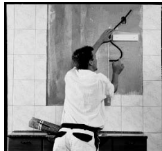
Mount a flex pipe in the wall from mirror to connection box.
